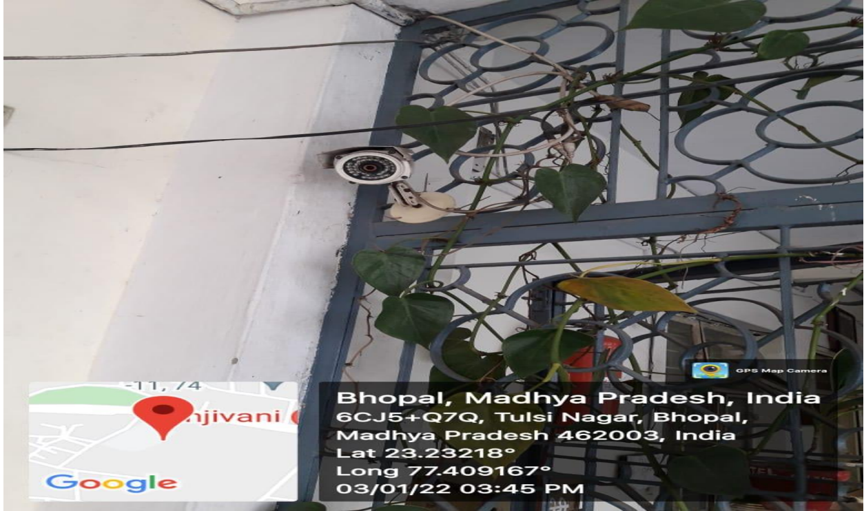
CCTV with in Premises
